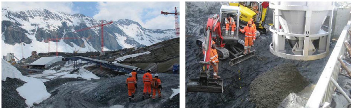
Figure 3. Project Linthal 2012. Left: material deposit and gravel plant (dry broken); right: dam concrete
